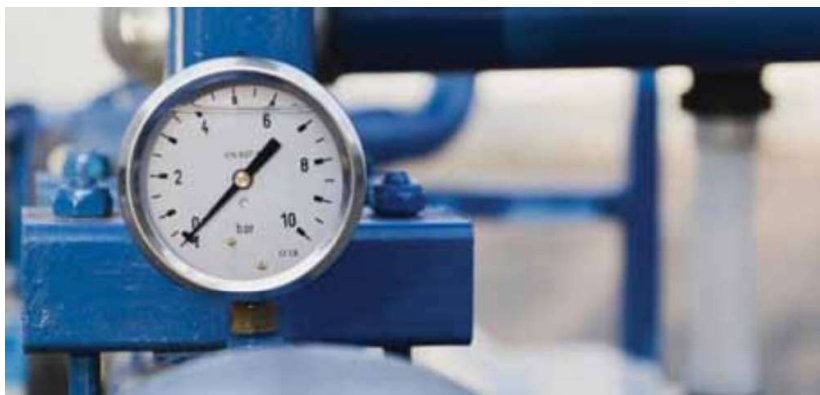
✧ Pressure drop measuring station.
